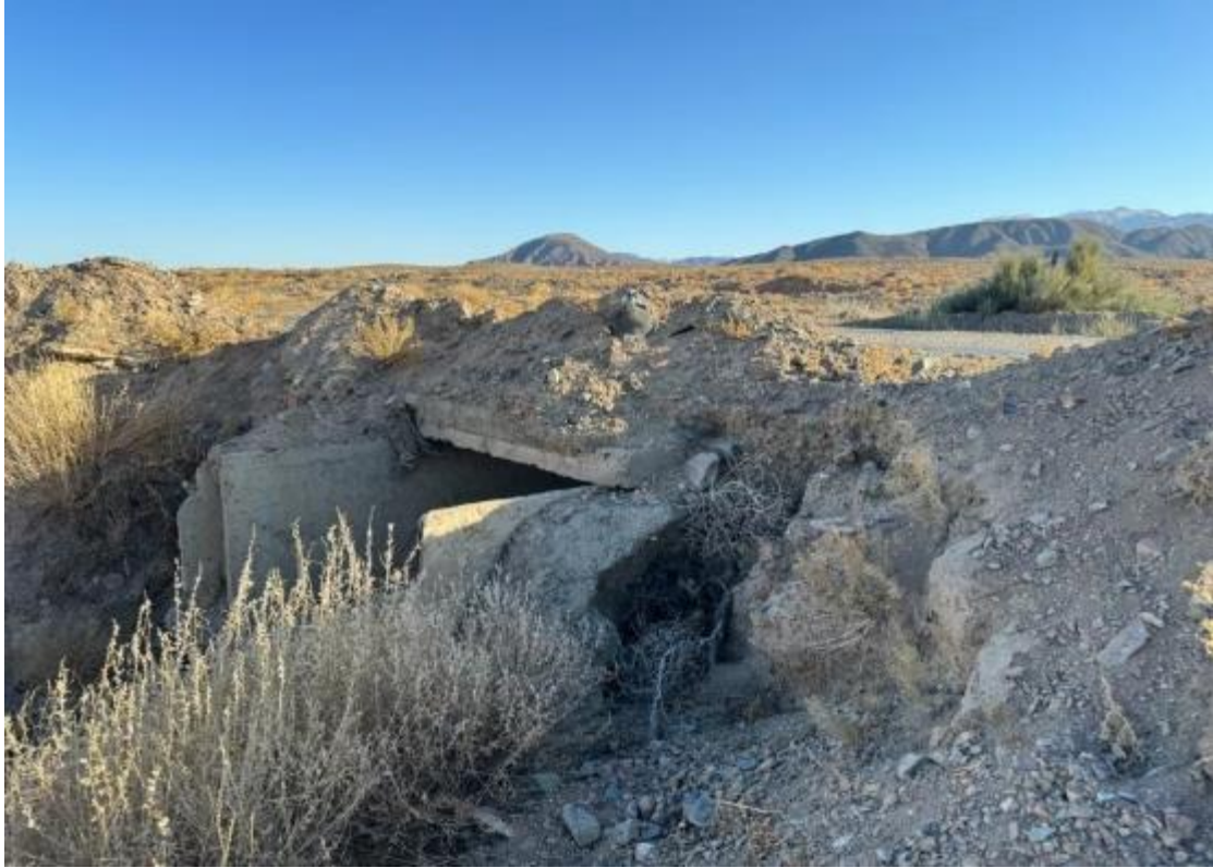
Photo 10. Condition of head/wing of water drainage structures at entrance. Soil erosion.
